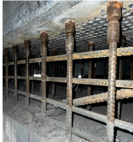
Figure 20. Surface between the first concreting phase and the second phase after hydrodemolition
