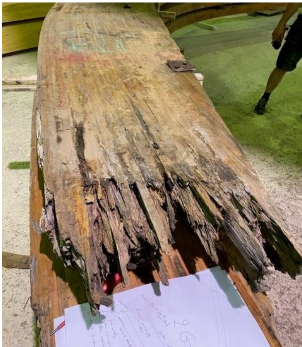
Figure 4. Degradation caused by water exposure
