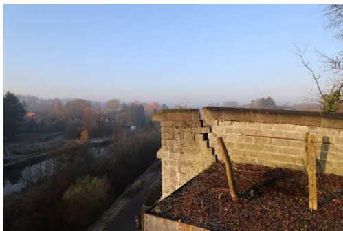
Figure 12: Side wall in P3 to rebuild
